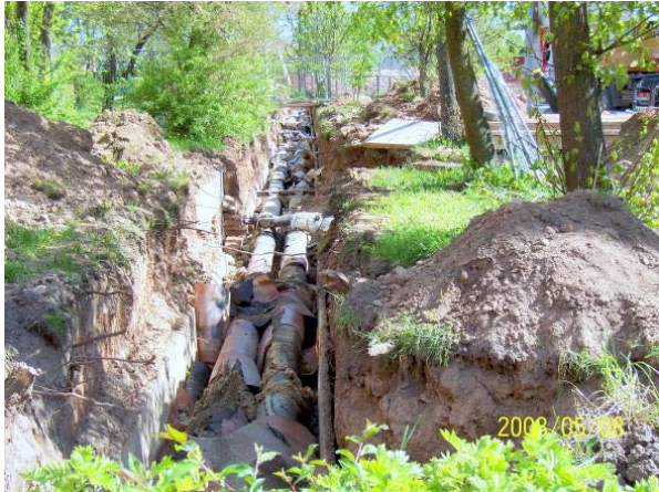
Figure 16 Old exposed pipelines
