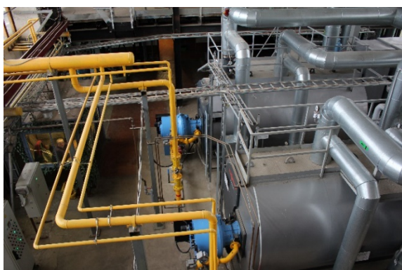
Figure 11 Old fossil fuel fired boiler
