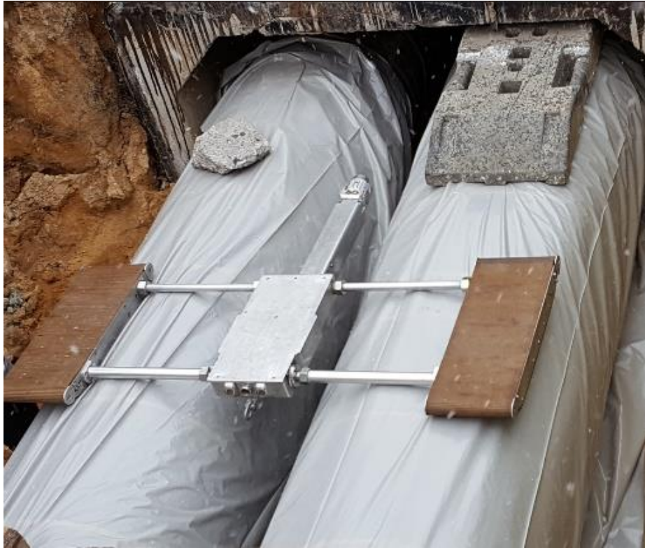
Figure 27 Visual inspection with the “Crawler Eye” of the German Institut für Angewandte Bauforschung Weimar gGmbH (Source: AGFW)
