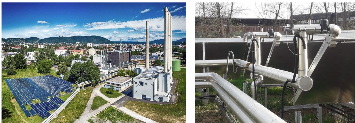
Figure 35: Solar thermal collector field in Graz, Austria, which feeds into the Graz DH network (Sources: left: SOLID; right: D. Rutz)
