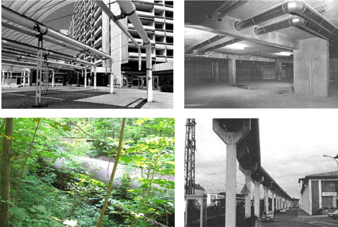
Figure 31: Examples of above ground and overhead pipelines (Source: AGFW, 1987)
