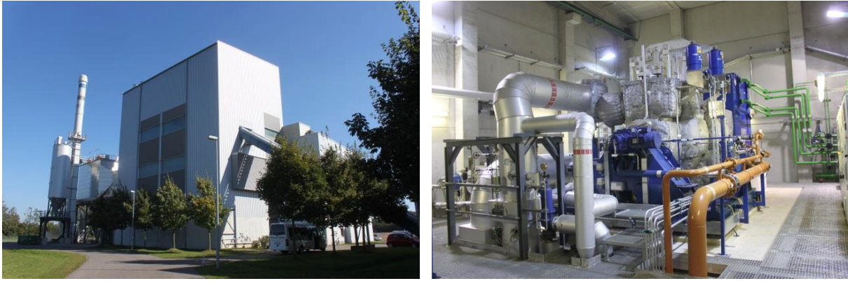
Figure 44: Wood chip fired CHP plant and its steam turbine of the Stadtwerke Augsburg Energie GmbH in Germany (capacity: 80,000 t/a wood chips; 7.8 MW el ; 15 MW th ) (Sources: D. Rutz)
