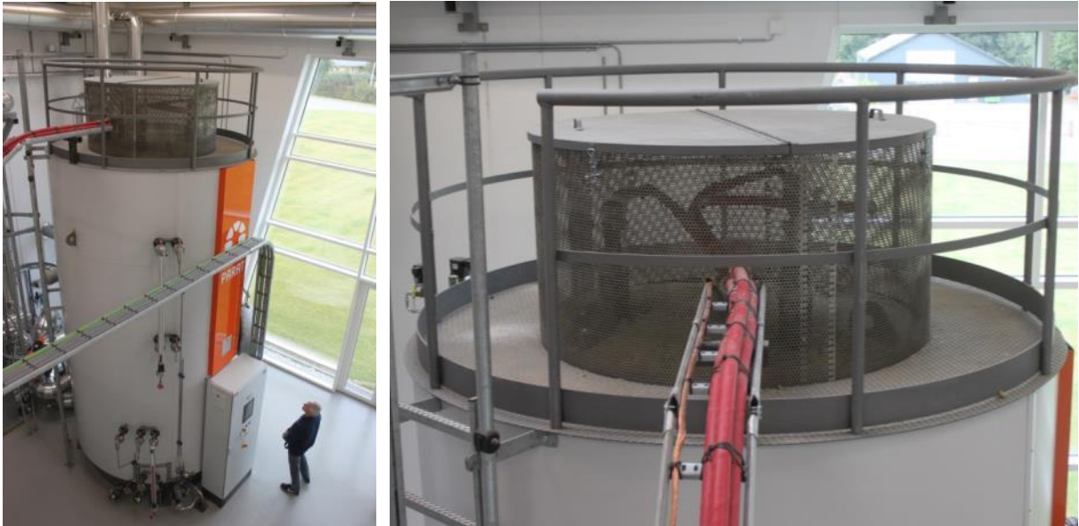
Figure 51: Electrode boiler of 10 MW and 14.4 m 3 capacity of the solar DH plant in Gram, Denmark (Source: D. Rutz)
