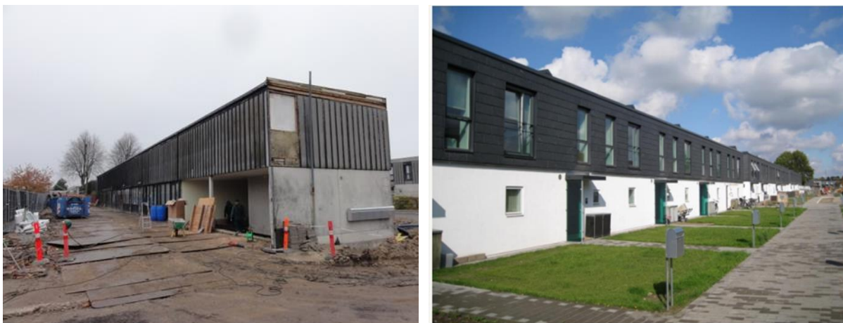
Figure 25: Buildings in Albertslund, Denmark before (left) and after (right) refurbishment (Source: COWI)
